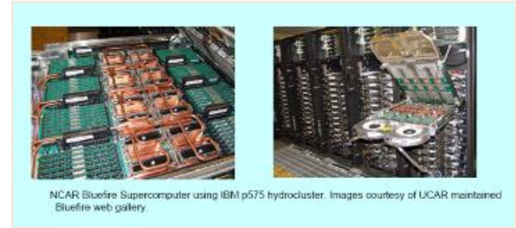
Liquid Cooling of Boards
