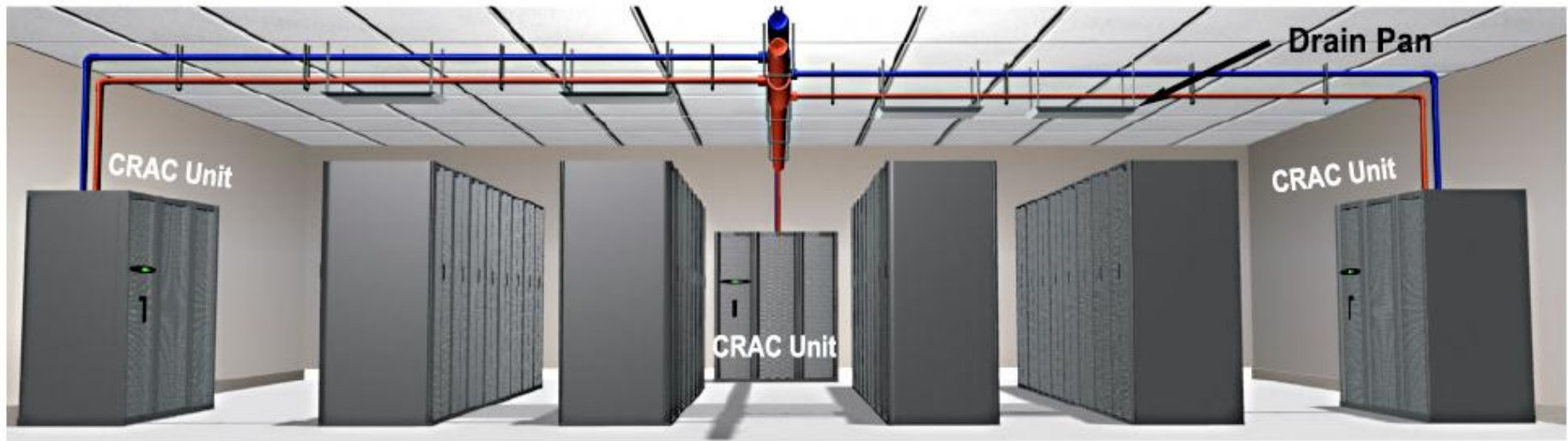
Figure 2 – Overhead piping with drain pan above racks.
